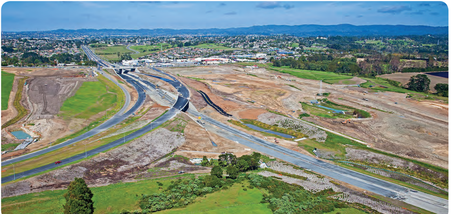
An aerial view of the new SH16 Hobsonville Road Interchange and SH18-SH16 flyover.
