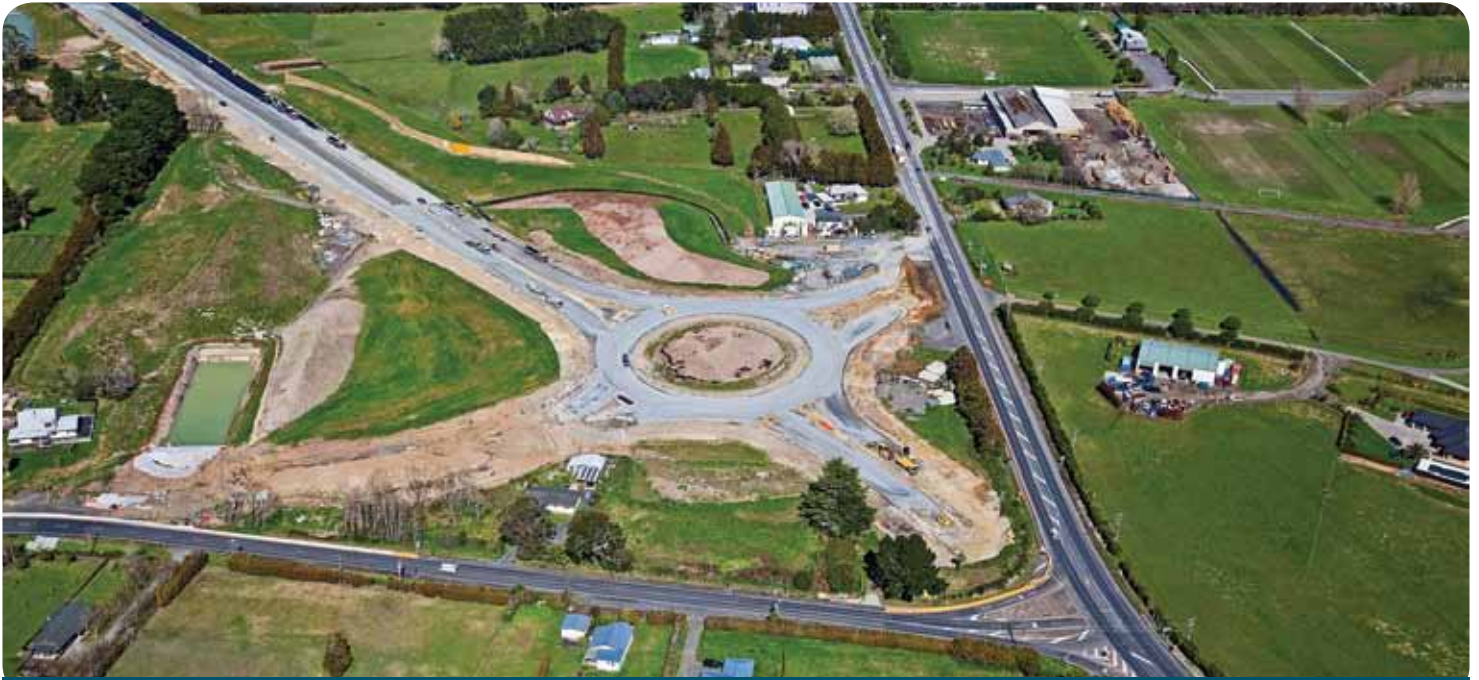
A birds eye view of the new Brigham Creek Extension and the roundabout that opens to traffic early next year.
