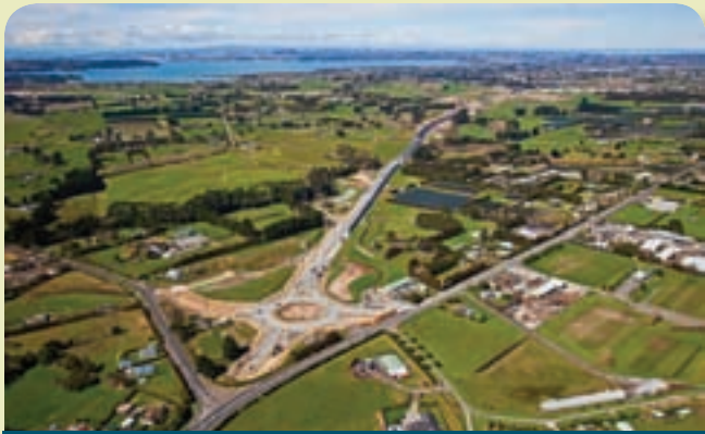
The path of the new SH16 Brigham Creek Extension is taking shape.
