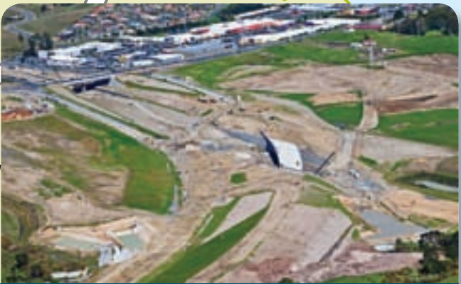
The SH18/SH16 Flyover is a vital link for motorists travelling between the west and the north shore.
