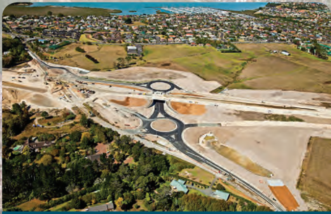
The new Brigham Creek Interchange with SH18 includes construction of three roundabouts along Brigham Creek Road.
