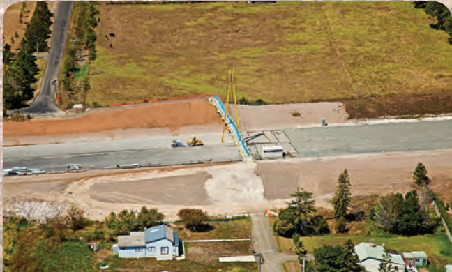
The iconic yellow Clarks Lane footbridge nears completion as the gateway to Waitakere City.
