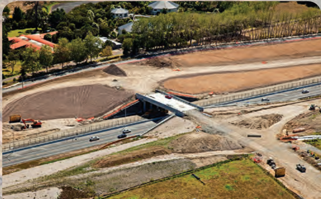
Squadron Drive Bridge will carry local traffic over the motorway when it is completed.
