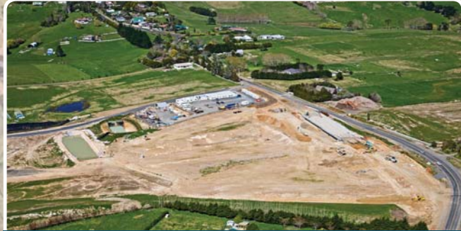
Trig Road Bridge will carry local traffic over the motorway when it is completed
