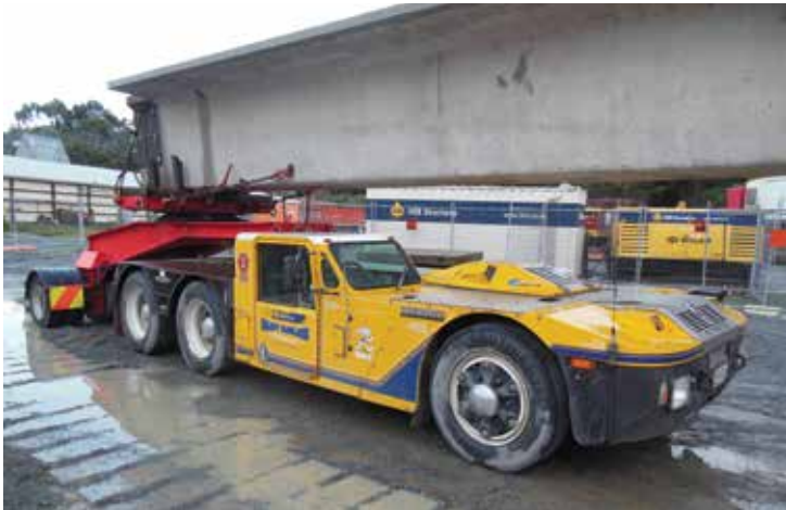
Each 31m beam is transported from Tauranga by road using a truck and a specialised vehicle called a jinker.
