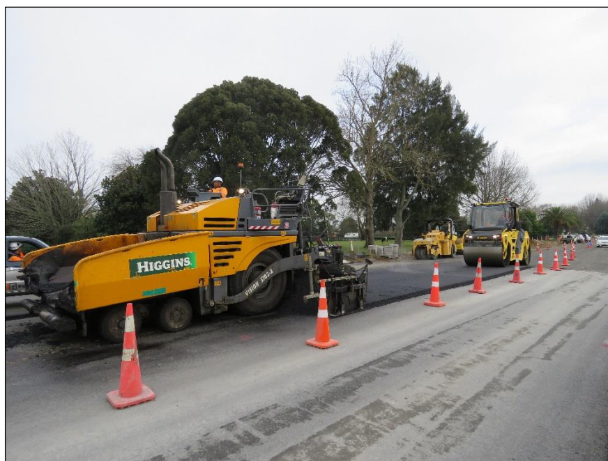
Multiple layers of asphalt are laid and compacted to create a smooth, lasting surface.
