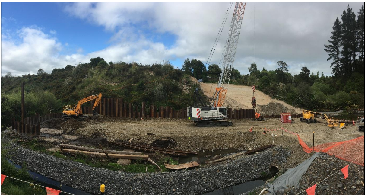
Sheet piles are installed to stabilise a gully bank prior to digging out wet material and installing a culvert.
