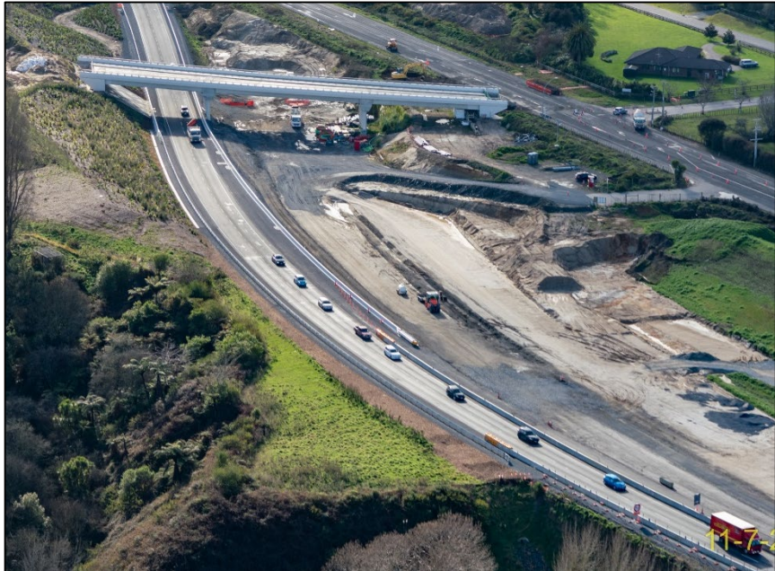
SH1 traffic flowing on the new lanes under the East West Link Bridge.
