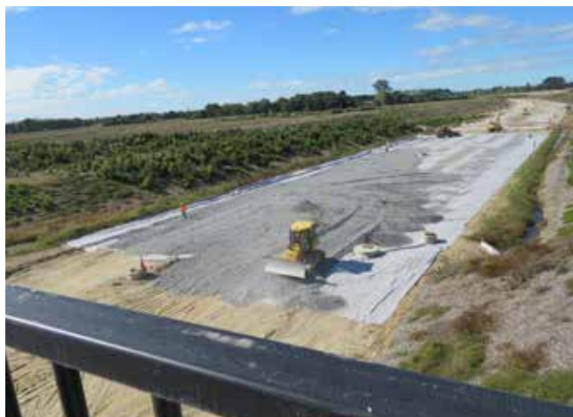
An extra layer of rock is laid at Ruakura to provide additional drainage.
