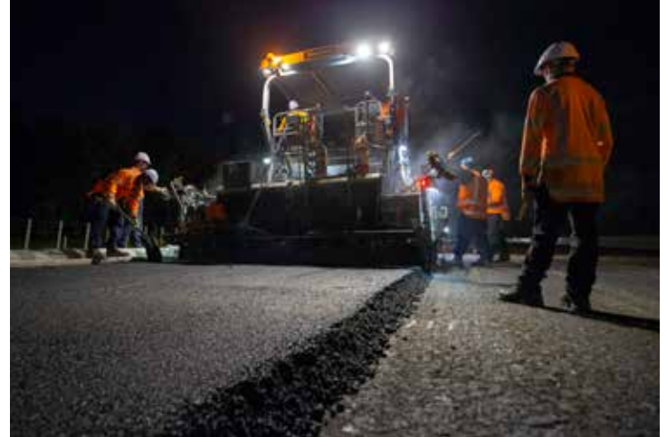
Trucks deliver the hot asphalt and tip it into the paver machine. The paver then distributes a continuous layer of asphalt onto the base of Hi-Lab rock.
