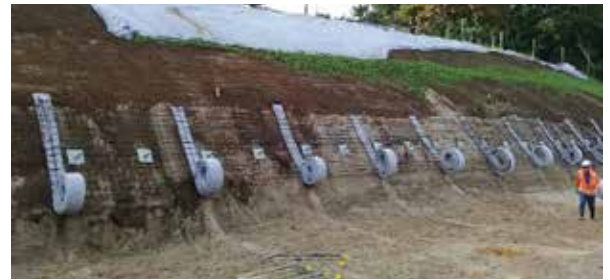
8-metre soil nails are placed between coils of drain. These drains unroll and extend as each new section of wall is shaped and nailed below this layer.
