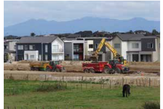
Earthworks in progress on the Resolution Drive Extension, with Tennille Street in the background.
