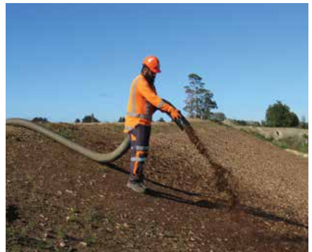
Compressed air is used to blow woodchip mulch into the slopes along the expressway embankments to prepare for planting.
