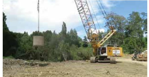
A large weight is used to form columns of rock under the ground to increase the strength of the soft gully soils.
