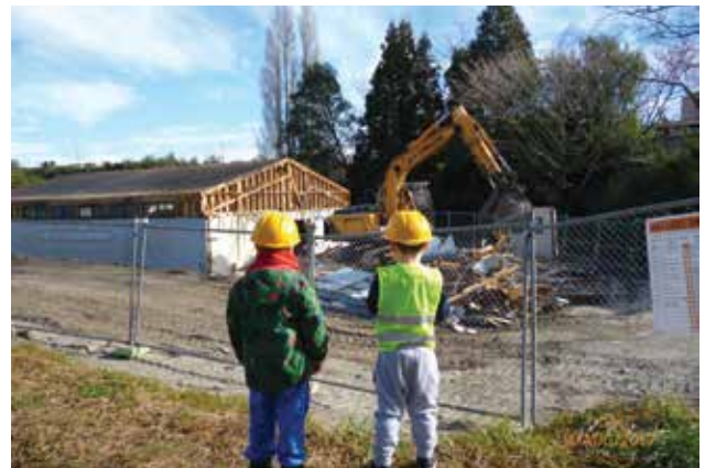
The demolition of the old Scout hall was exciting to watch for these local children.
