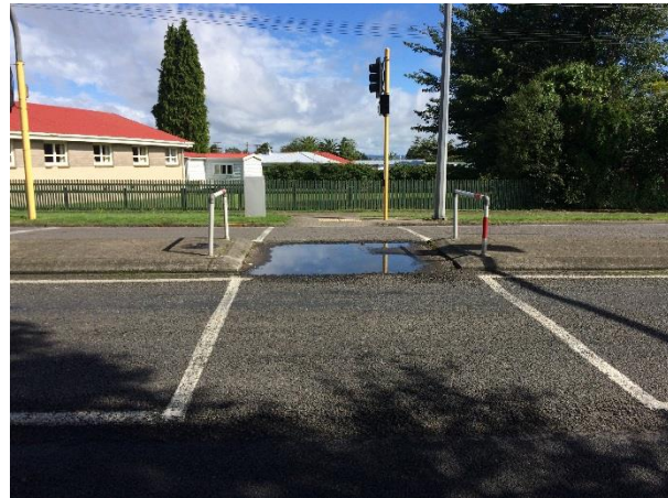
Figure 7-8: Ponding at the Coulter Road pedestrian crossing
