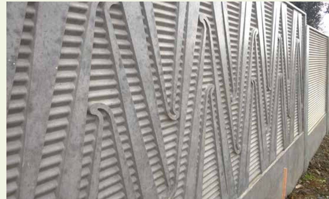
Kirkbride Road/State Highway 20A, Auckland - fine detail on noise wall alongside shared path
