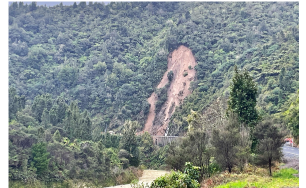
Above: A slip through SH2 Waioeka Gorge as a result of recent rain.
