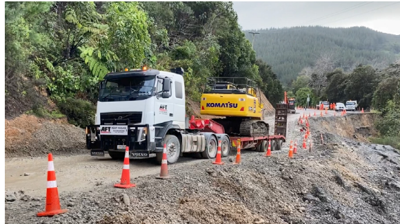
Above: A truck and trailer unit moves through Kopuaroa Hill (permitted 7am to 7pm only).
