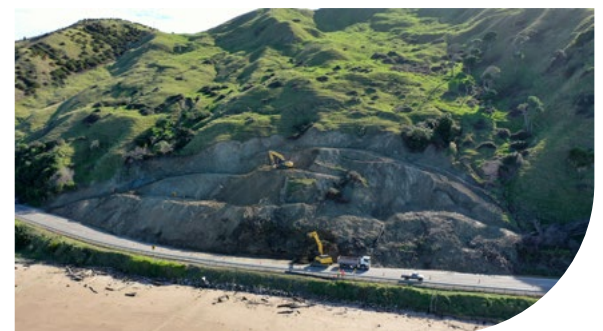
Above: Drone shot of work to clear the Makorori Slip (Photo: Ben Cowper)
