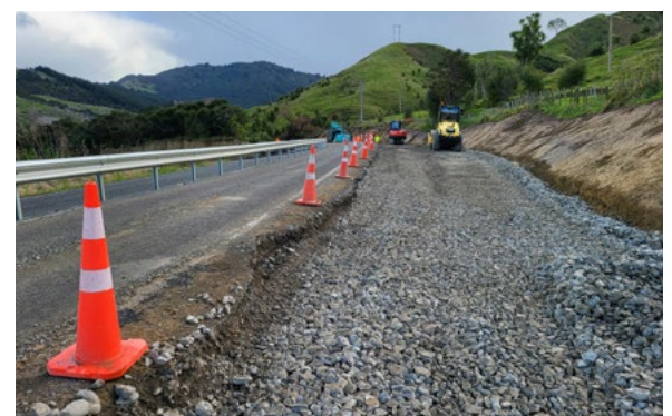
Above: Also north of Tokomaru Bay, the hillside has been excavated and the state highway shifted over to avoid a drop-out alongside the Mangahauini River
