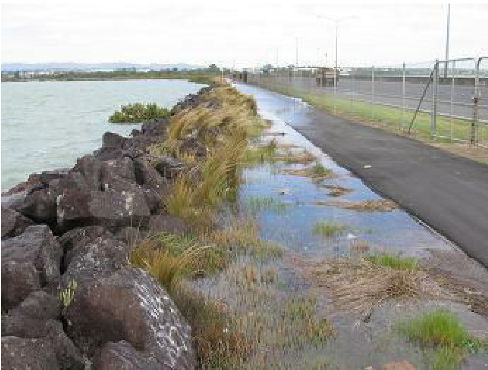
Figure 5.7: Landward side of causeway looking west with minor flooding from high spring tide
