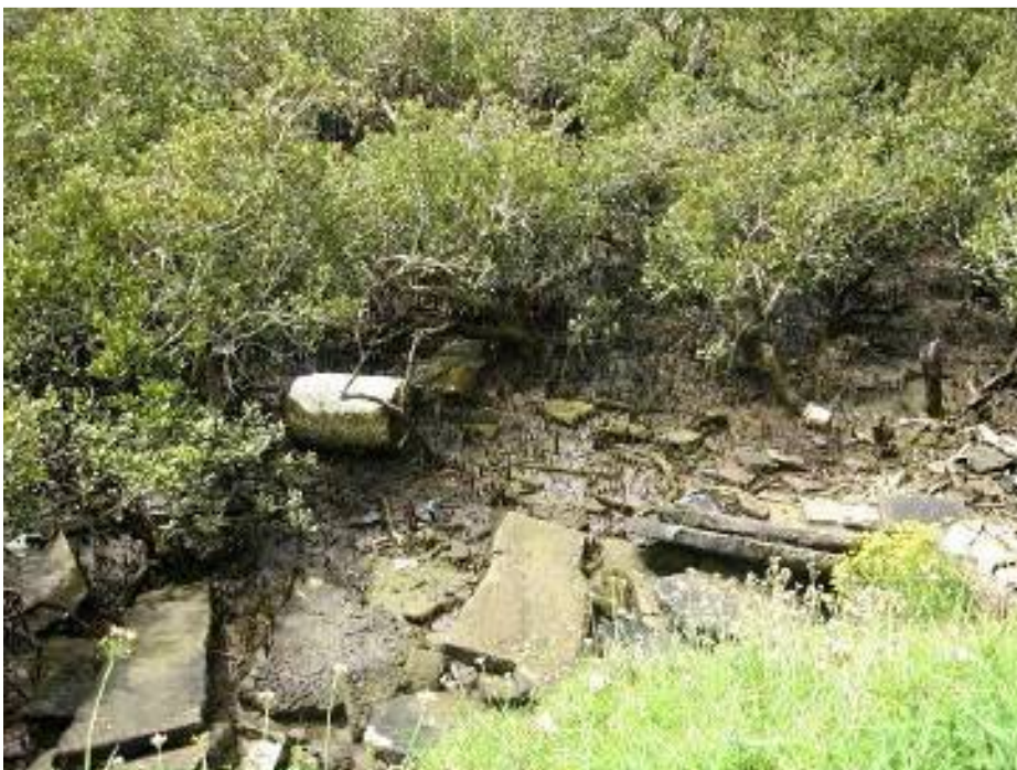
Figure 5.2: Existing outlet at 675 diameter culvert at the proposed site for Jack Colvin Wetland
