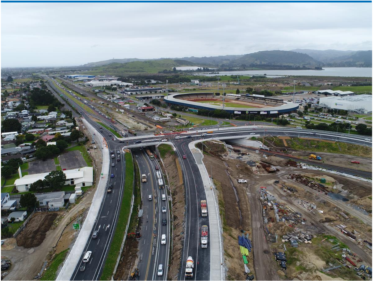
Partial opening of the new SH2/29A Te Maunga interchange at the Baypark end of the project in July.
