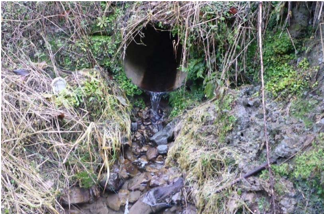
Figure 4.4 – Fish barriers on small intermittent streams from the current SH3. Site Ea1/Ea2 (top) site Ea21 (bottom) (1 August 2017). Limited fish habitat upstream of these barriers reduces their overall effect on fish populations.
