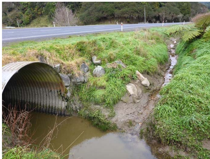
Figure D 32 – Mangapepeke Stream culvert under the current SH3 north of Mt Messenger, August 2017. This site is not affected by the Project.
