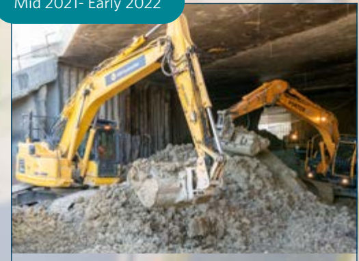
The big dig started in mid-2021 and over the course of many months (including a COVID-19 lockdown), 16,000m 3 of material - the equivalent of 6.5 Olympic sized swimming pools - was removed. The material was sent to a cleanfill site so that it can be recycled and reused.
