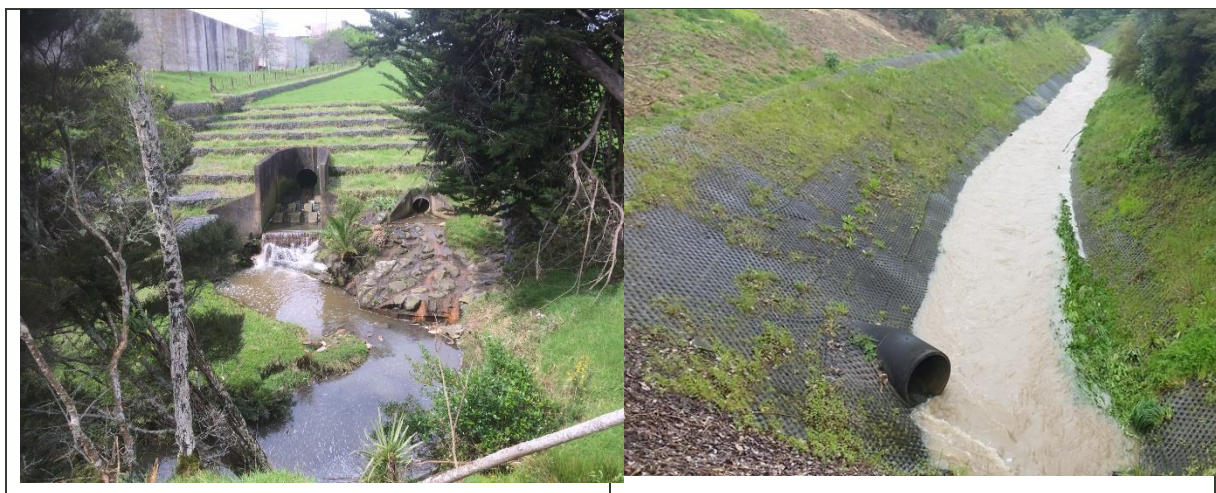
Figure 21 Existing erosion projection at Outfall Structure OF12, and armoured modified watercourse downstream of OF12.
