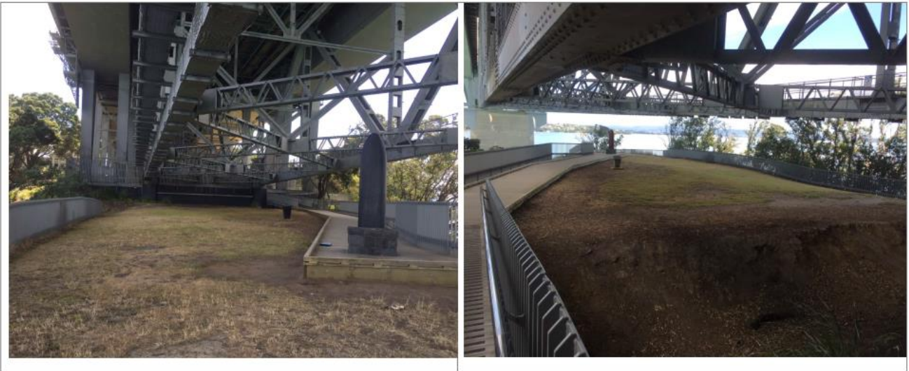
2 February 2021. Te Onewa Section; LHS – view to north towards North Anchorage; RHS – View to south from trench adjacent to North Anchorage showing Waitematā soils.
