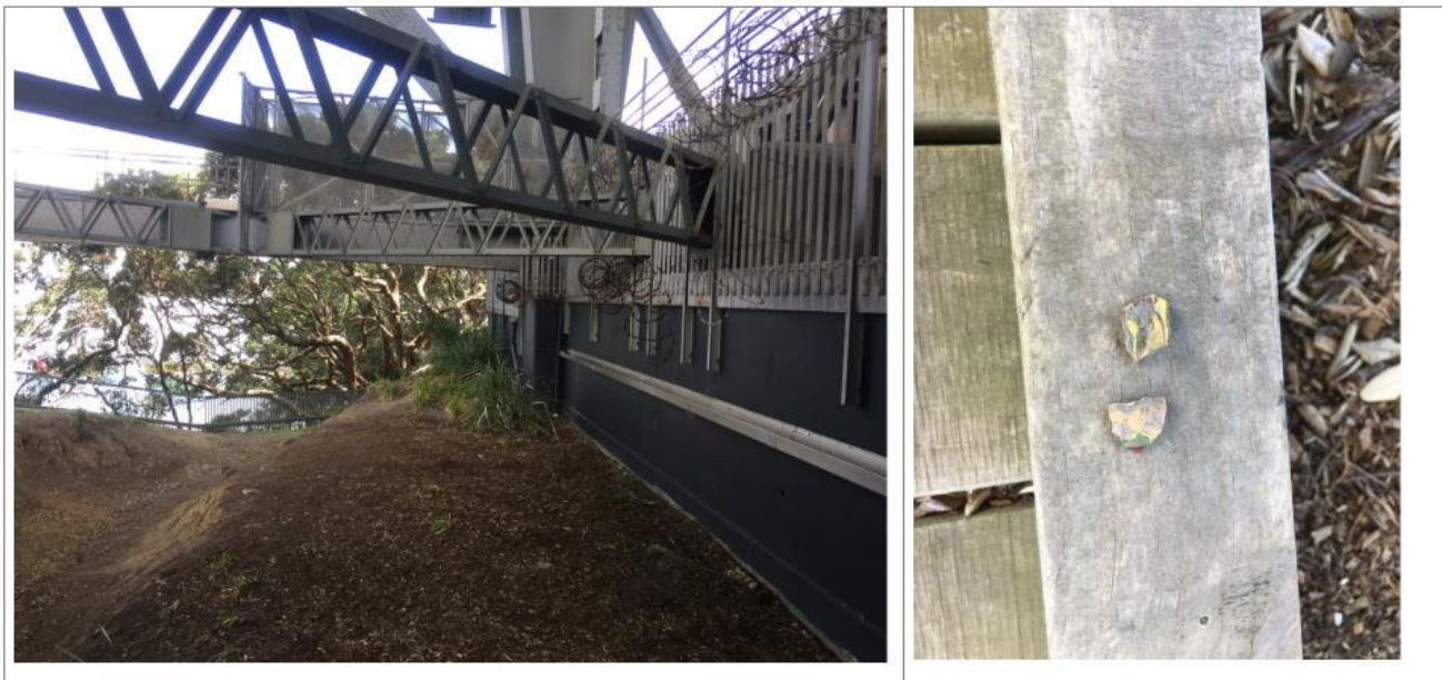
2 February 2021. Te Onewa Section; LHS – view to west from Anchorage; RHS – Paint flakes
