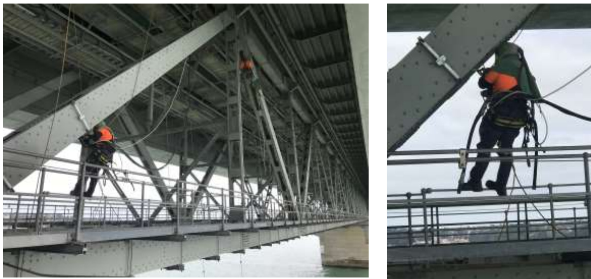
Fig 1.1 and 1.2 Abrasive Blaster operators spot blasting on diagonals on each side of post 5.3 on eastern side of bridge
