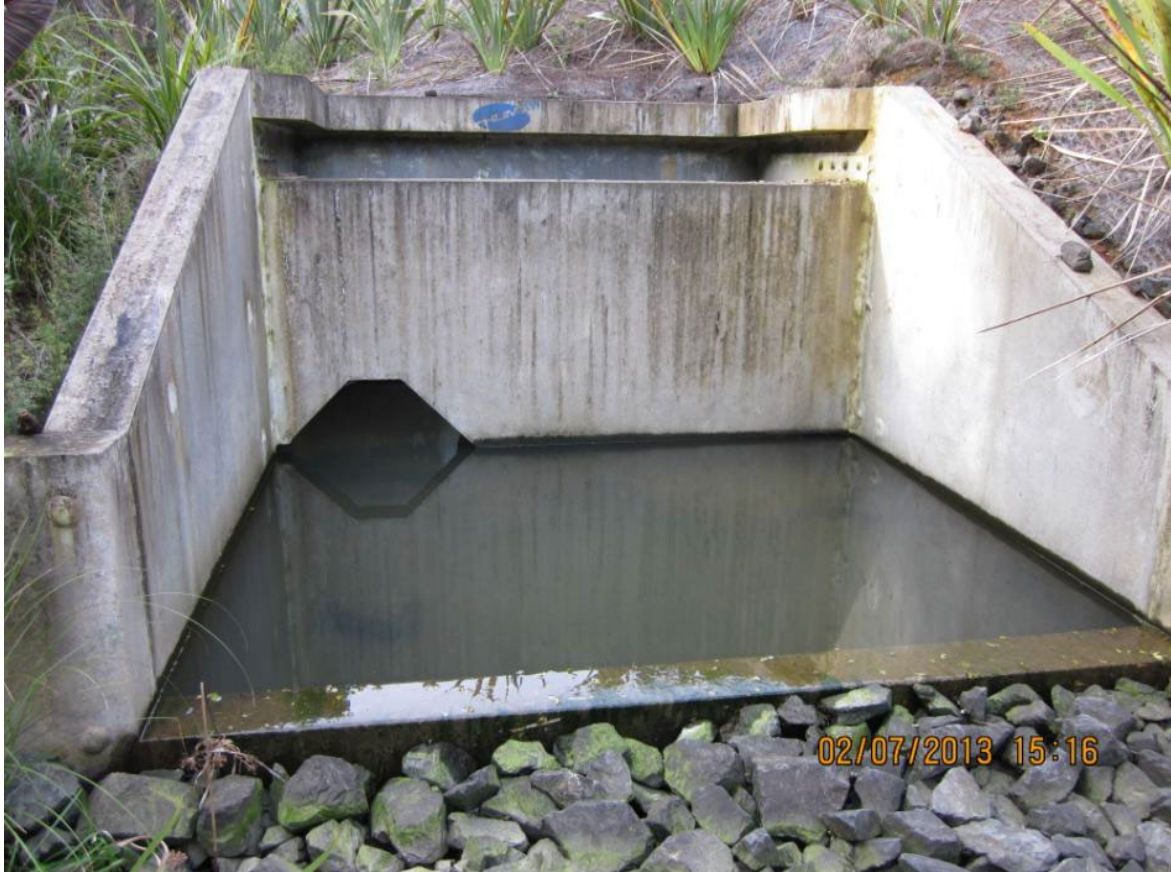
Photo 1 - Impact basin on NGTR Otanerua Wetland outfall
