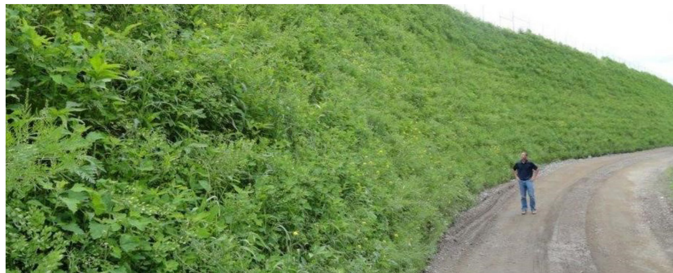
MSE Retaining wall with a soil and vegetation system integrated. No exotic species with potential to invade areas of native bush.
