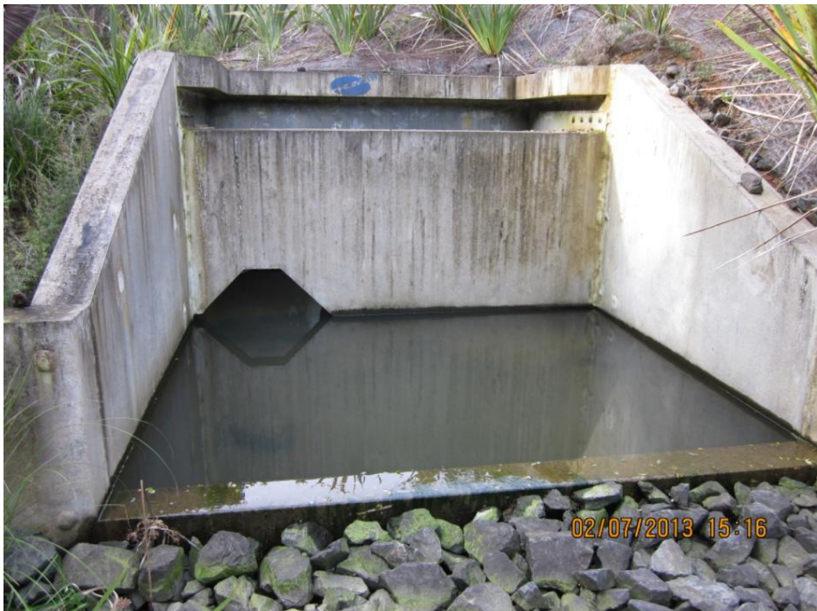
Photo 1 – Impact basin on NGTR Otanerua Wetland outfall
