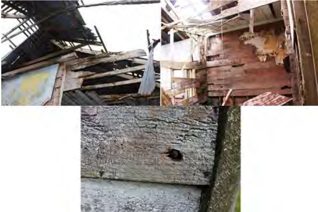
Figure 83 – Examples of the poor condition of Woodthorpe House
