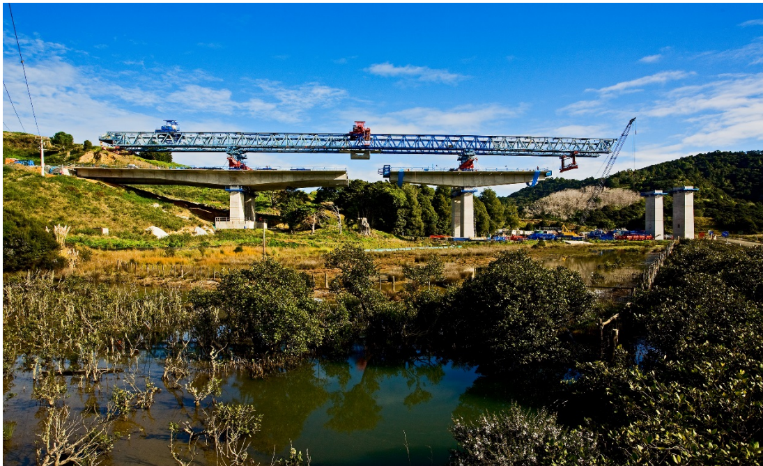
Figure 11 - A launching gantry placing segmental box girder sections on the Waiwera Viaduct
