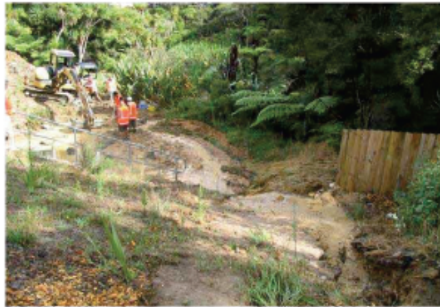
Sediment Discharge as a Result of Not Protecting the Watercourse
