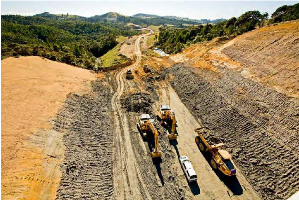
Figure 5-1: Bulk earthworks on Northern Gateway Toll Road, similar to proposed earthworks through the commercial plantation forestry
