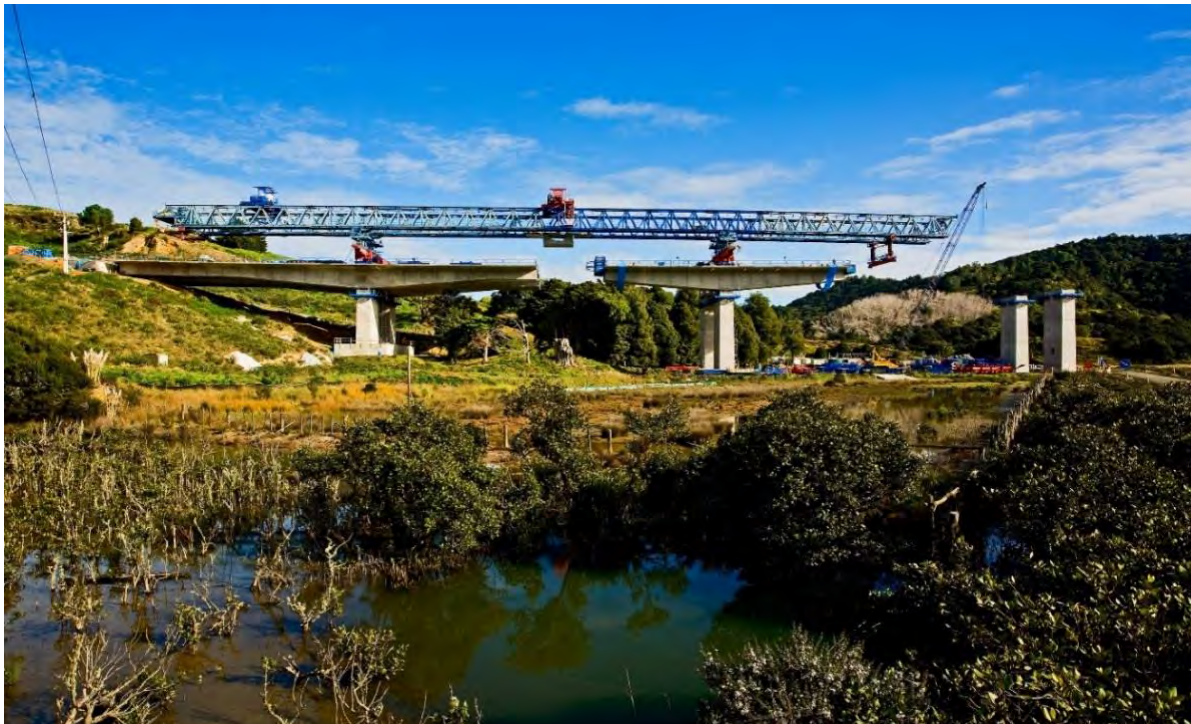
Figure 5-7: A launching gantry placing segmental box girder sections on the Waiwera Viaduct
