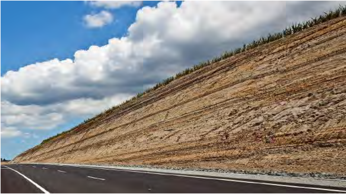
Figure 4-7: Indicative cut face batter (possible for cuts within the plantation forestry area)
