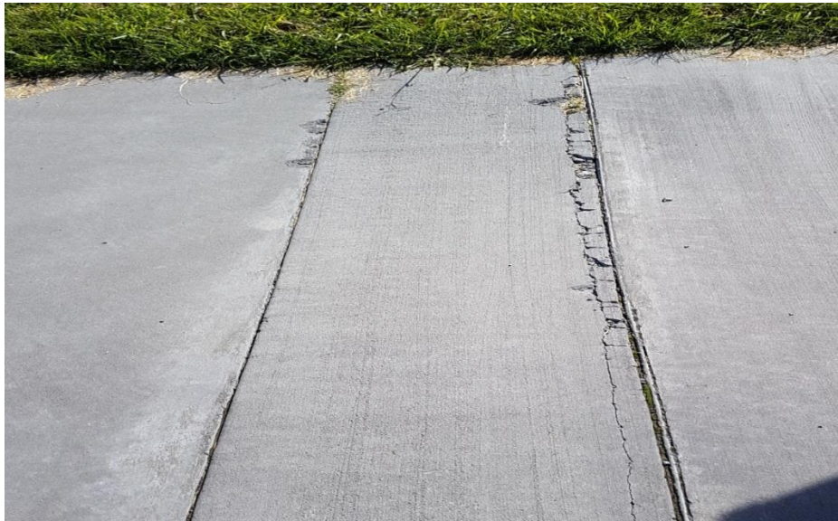
Figure 15: Surface defects at path joins with steel strips
