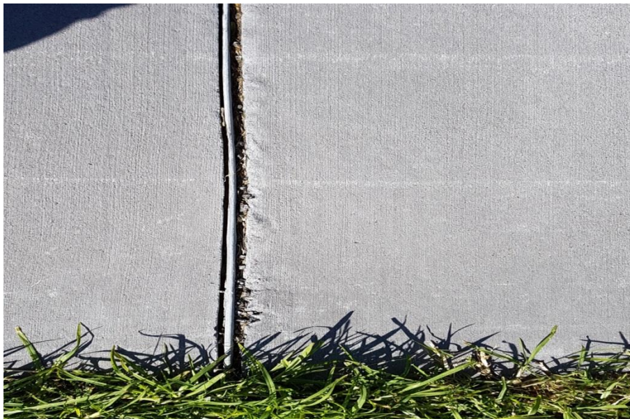
Figure 14: Surface defects at path joins with steel strips
