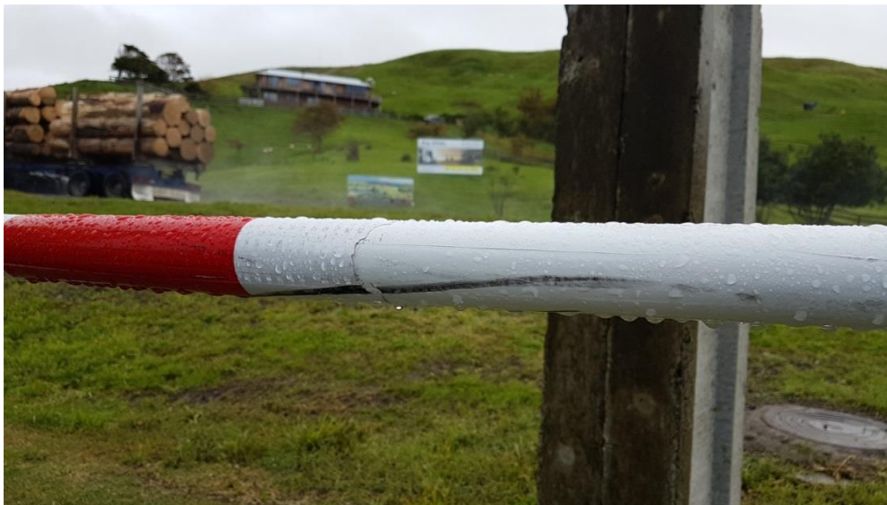
Figure 5: Width restrictor evidence of being struck
