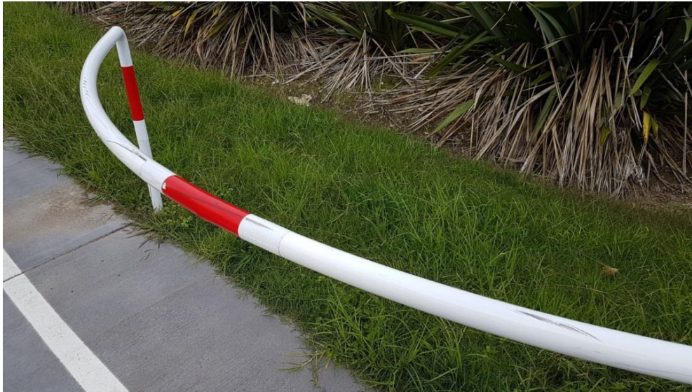
Figure 4: Width restrictor evidence of being struck
