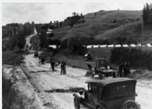
Road construction between Wellsford and Te Hana. c. 1920s. Photographer unidentified. Ref: PAColl-6181-41, Alexander Turnbull Library.
