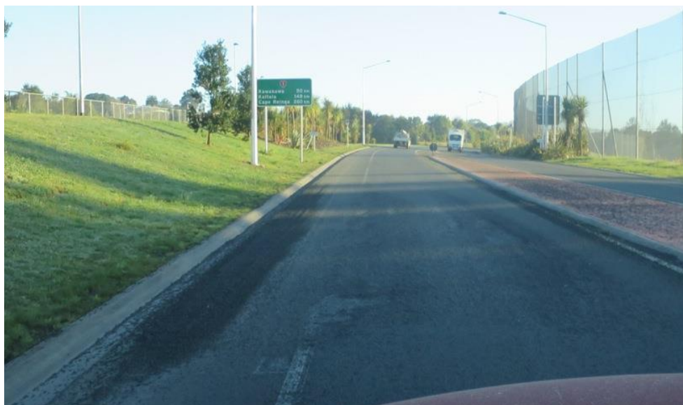
Figure 7: Kamo Bypass pavement deterioration
