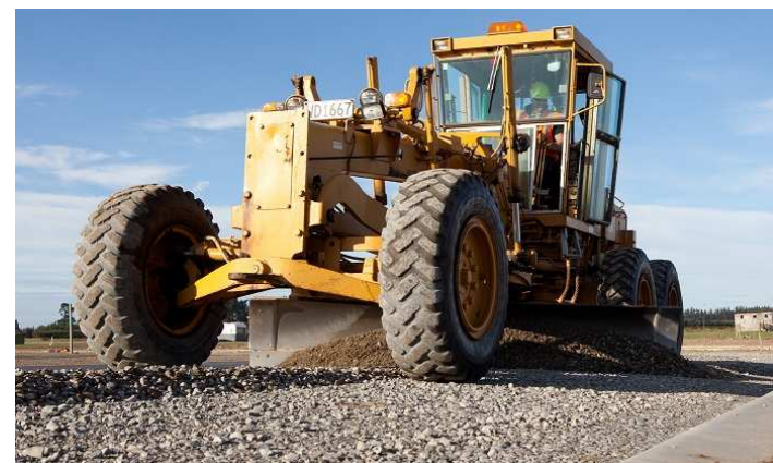
A grader is one of the pieces of machinery you will see in use on Johns Road.
