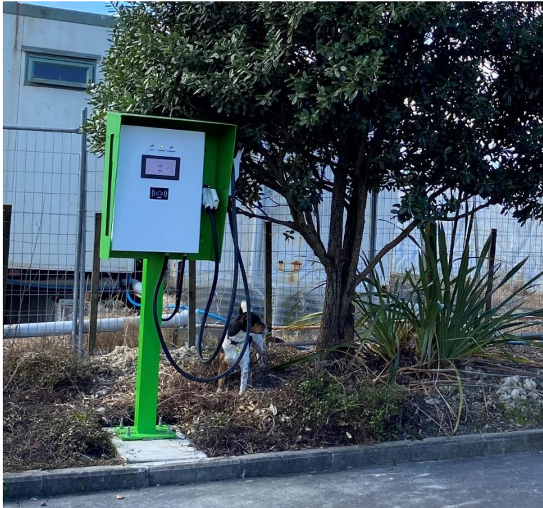
new charger on left, installed adjacent to original charger and fuse box
