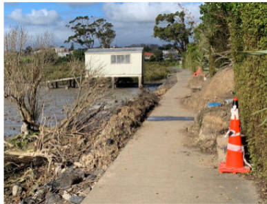
Landslip, no prior warning
