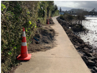
Landslip, no prior warning
