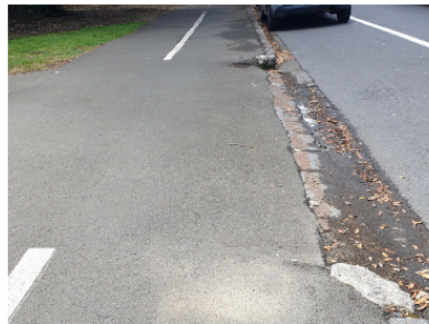
Unavoidable tipping danger caused by a wide kerb drop. This creates a lane less than 1m. A bit of paint here is needed to alert wider cycles.
