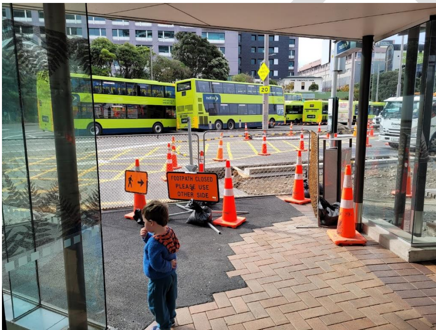
Figure 73: Temporary traffic management at Wellington Railway Station bus interchange. Source: Lorelei Schmitt.
