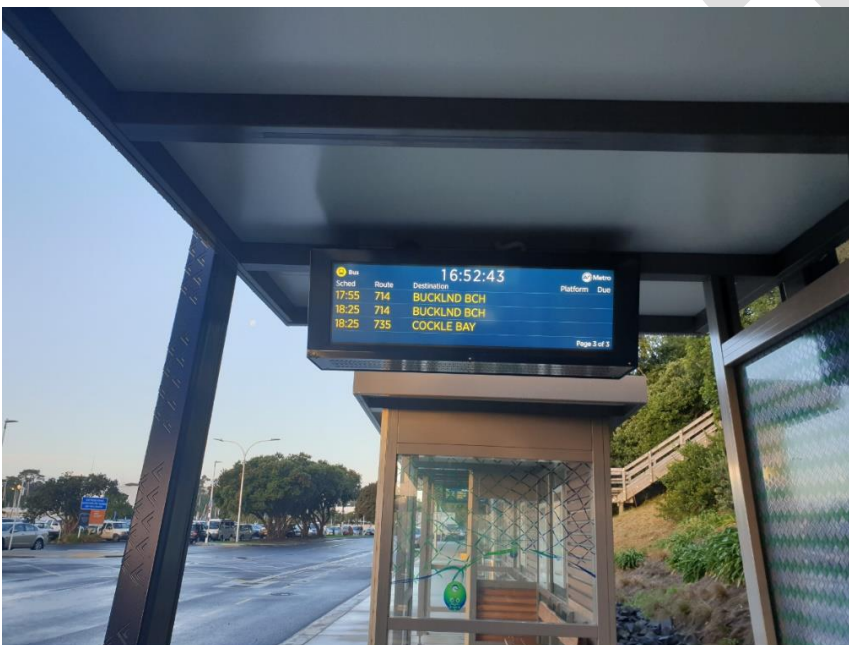
Figure 45: Real-time sign incorporated into a shelter. Source: Flow Transportation Specialists.
