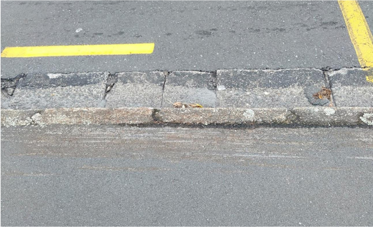
Figure 27: Damage to kerb and footpath from bus scraping associated with inadequate ground clearance (Source: Lorelei Schmitt)
