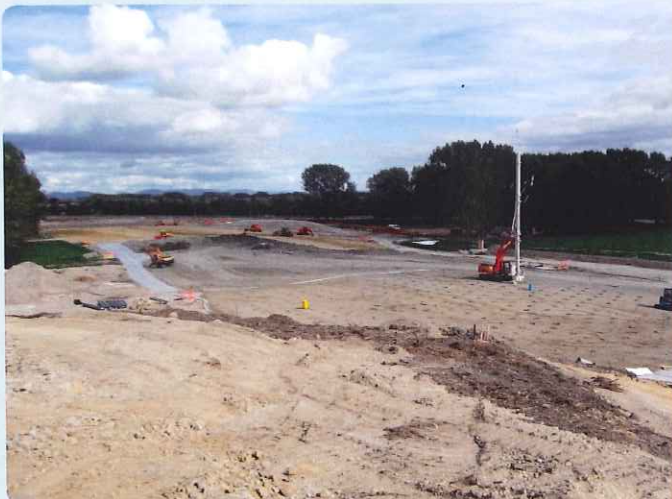
Earthworks in the region of 400m north off Glen Murray Road showing wick drains.
