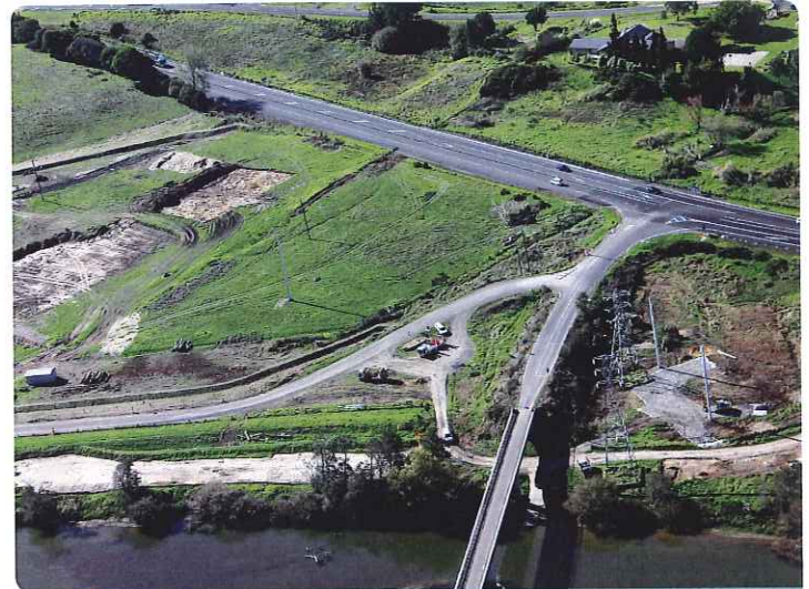
Aerial view of future Rangiriri Interchange, with Transpower pylon relocation works underway on bottom right hand side.
