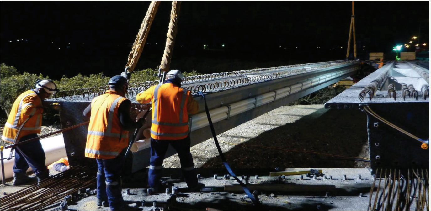
The new Henderson Creek Bridge currently under construction. Traffic will be switched onto this in mid-November
