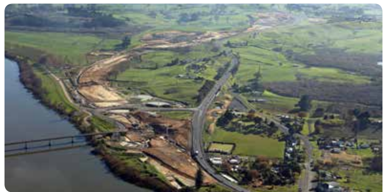
The southern start of the Rangiriri section looking north from the Waikato River
