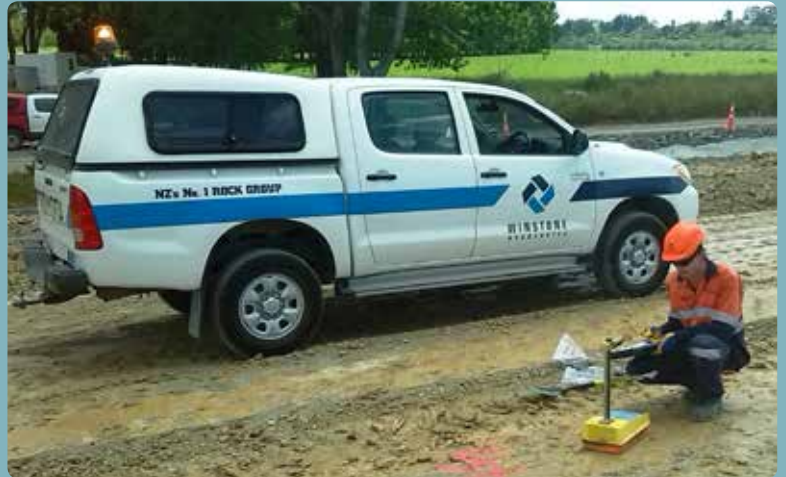
Laboratory manager using a Nuclear Densometer on site to determine density and moisture of the ground
