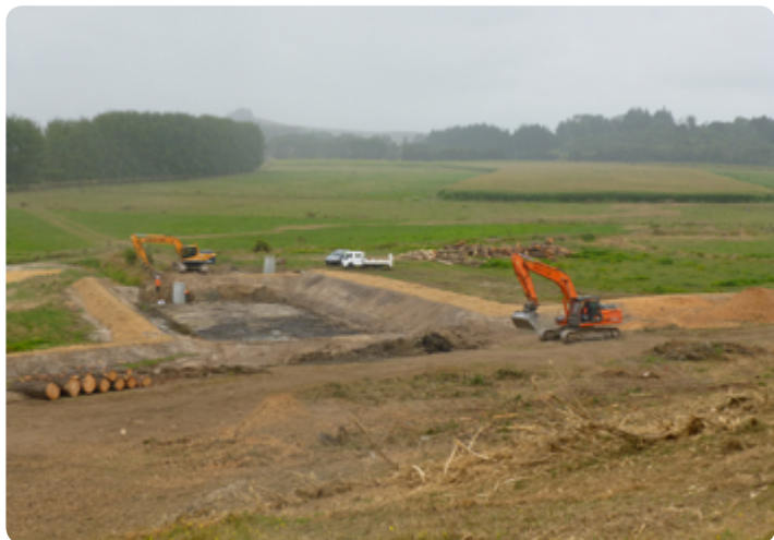
Construction of one of the earth bunds as part of the environmental controls for the project
