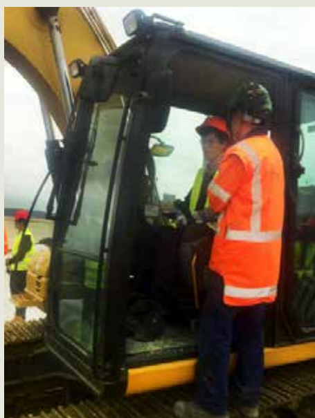
Massey High School Construction Trades Academy students experienced the driver's seat and GPS equipment in a stationary excavator on site, with guidance from Kerry, Causeway Alliance Leading Hand (orange jacket).
