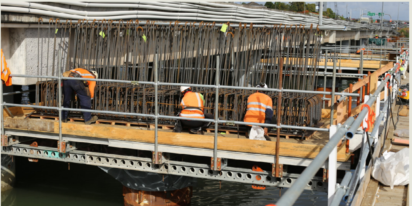
Photo by Colin Battley shows the temporary staging platform (right) for workers, SH16 eastbound on the left behind the barrier, and Causeway Alliance workers placing steel reinforcing bars to create the inside structure of the first of seven vertical crossheads.
