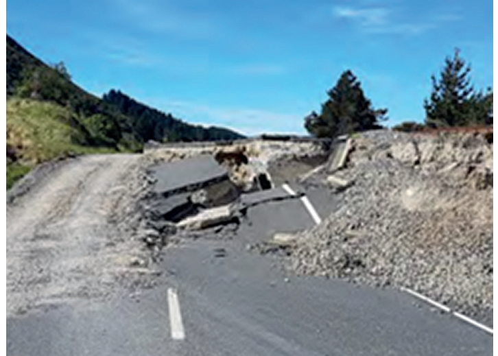
Fault rupture damage at Waipapa Bay, north Kaikōura coast
