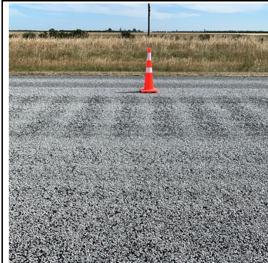
Corrugations in the right half of the lane after application of the grade 4 chip. Taken at 1620h.
