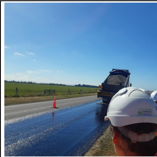
1 st coat of emulsion complete, applying grade 6 chip to left half of lane.
