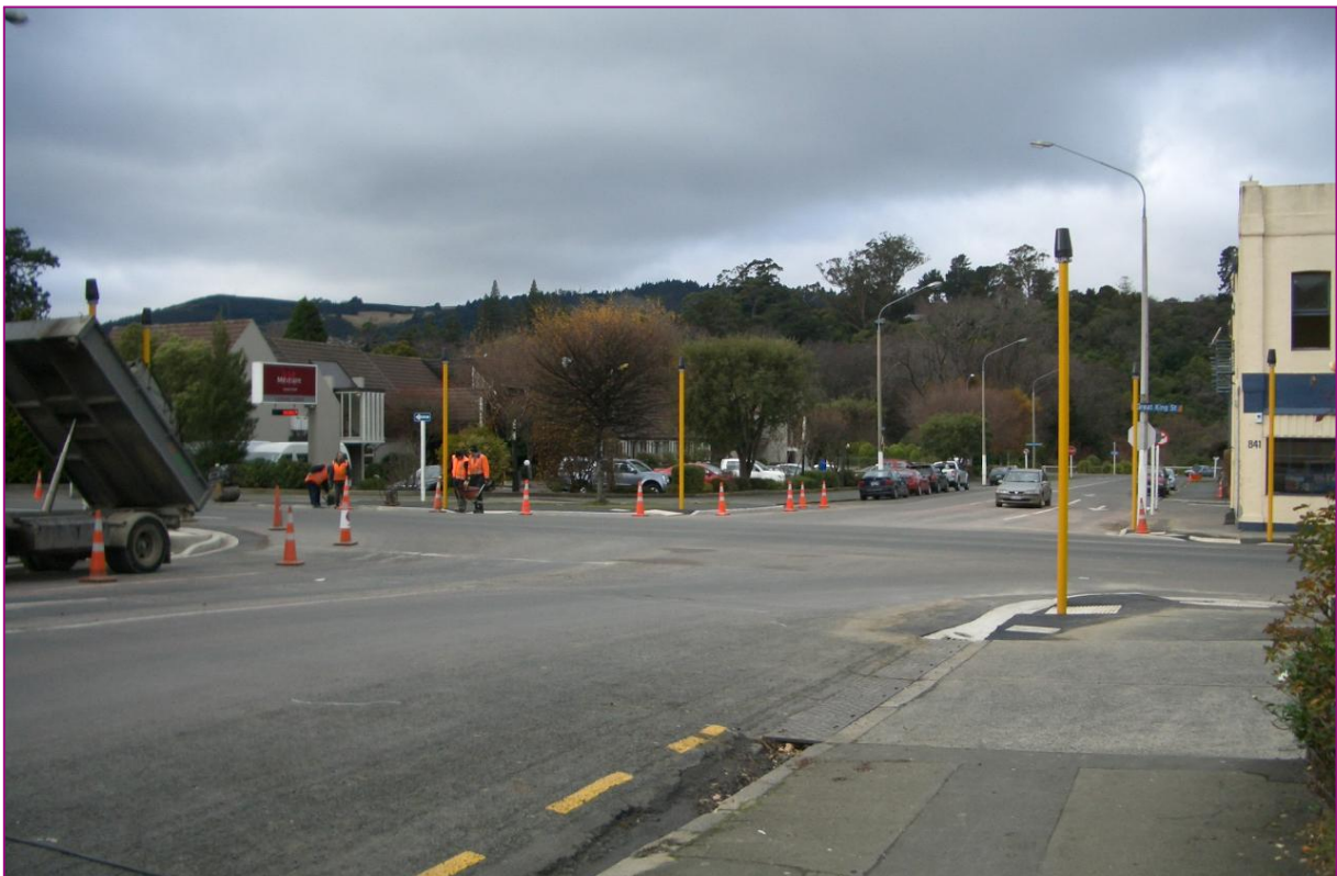
Figure 3 View of Duke Street Intersection from Southwest Corner (Mercure Hotel Visible on the Left)
