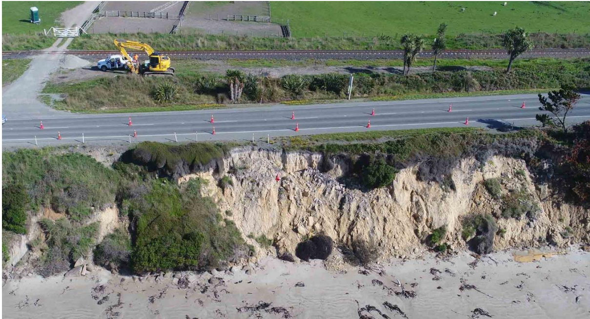
Figure 7: Cliff erosion State Highway 1 (Katiki Beach North Otago)
