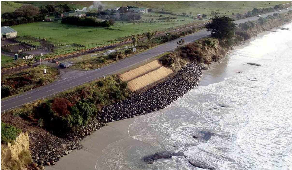
Figure 8: Rock armoring of cliff base and extension as reef into sea to break wave energy State Highway 1 (Katiki Beach North Otago)
