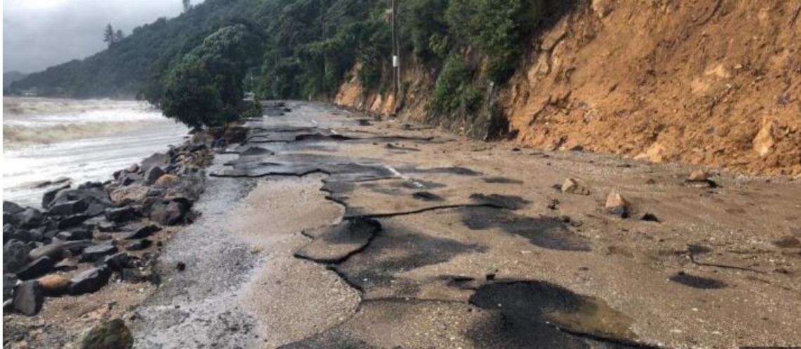
Figure 9: State Highway 25 (Firth of Thames Coromandel) coastal damage
