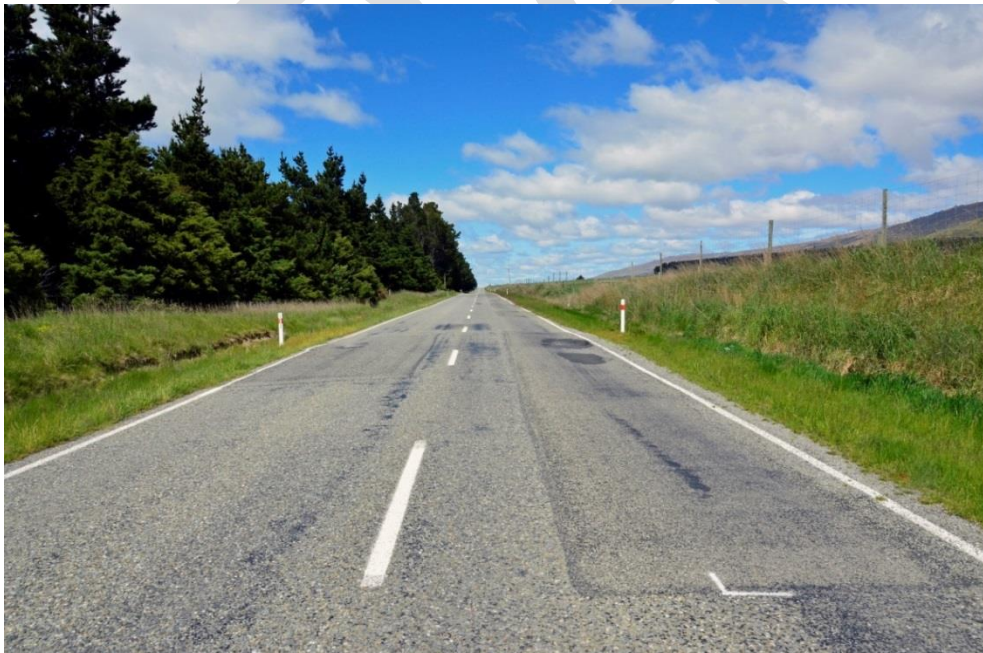
Evidence of poor road-side drainage.
