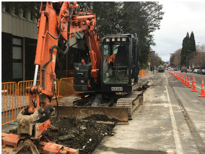
Kerb realignment work to create a bus stop bay on the new cycle lanes along SH1 on Cumberland Street south outside the University near St David Street
