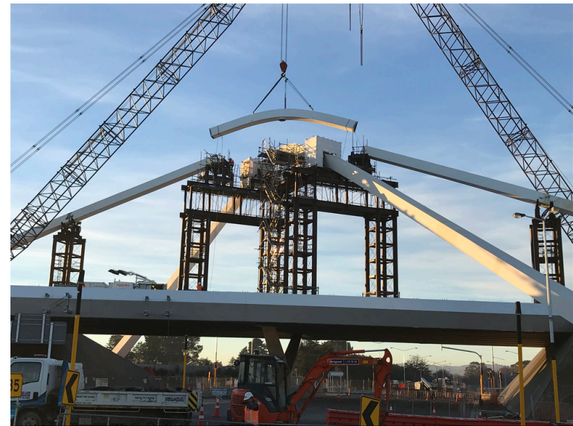
The top piece of the gateway arches going into place: Installation of gateway arches at intersection of Russley Road and Memorial Avenue in Christchurch
