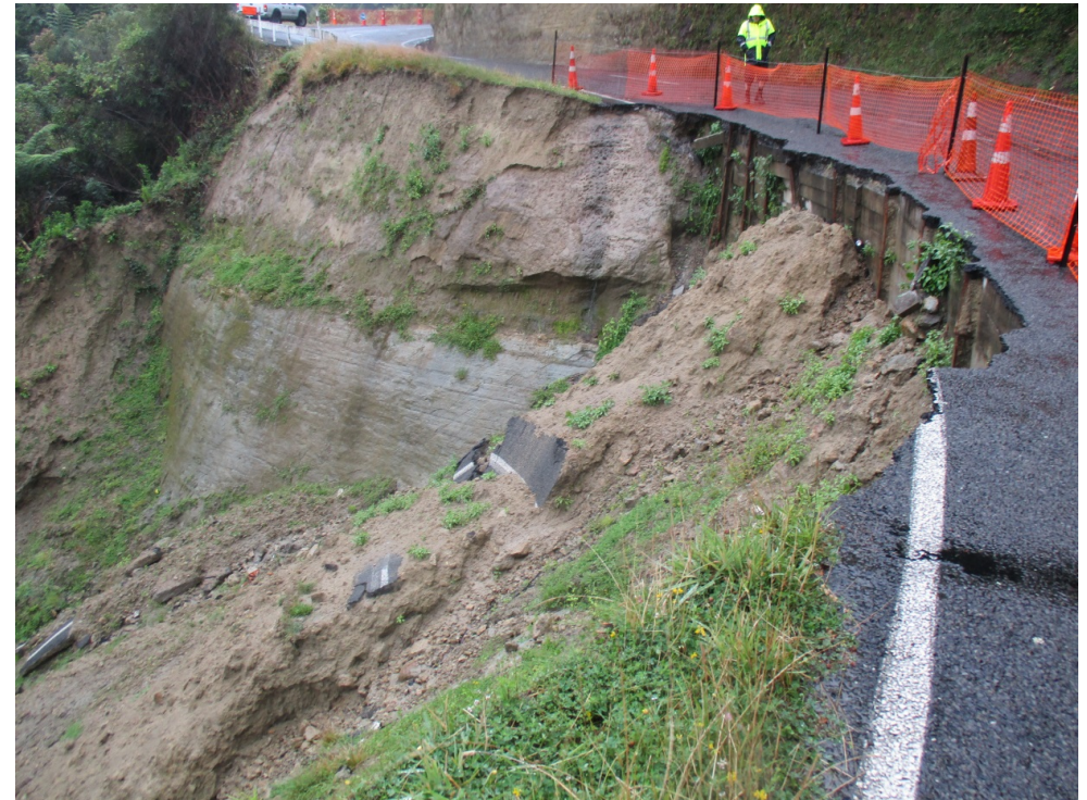
SH43 Pohukura Saddle Underslip
